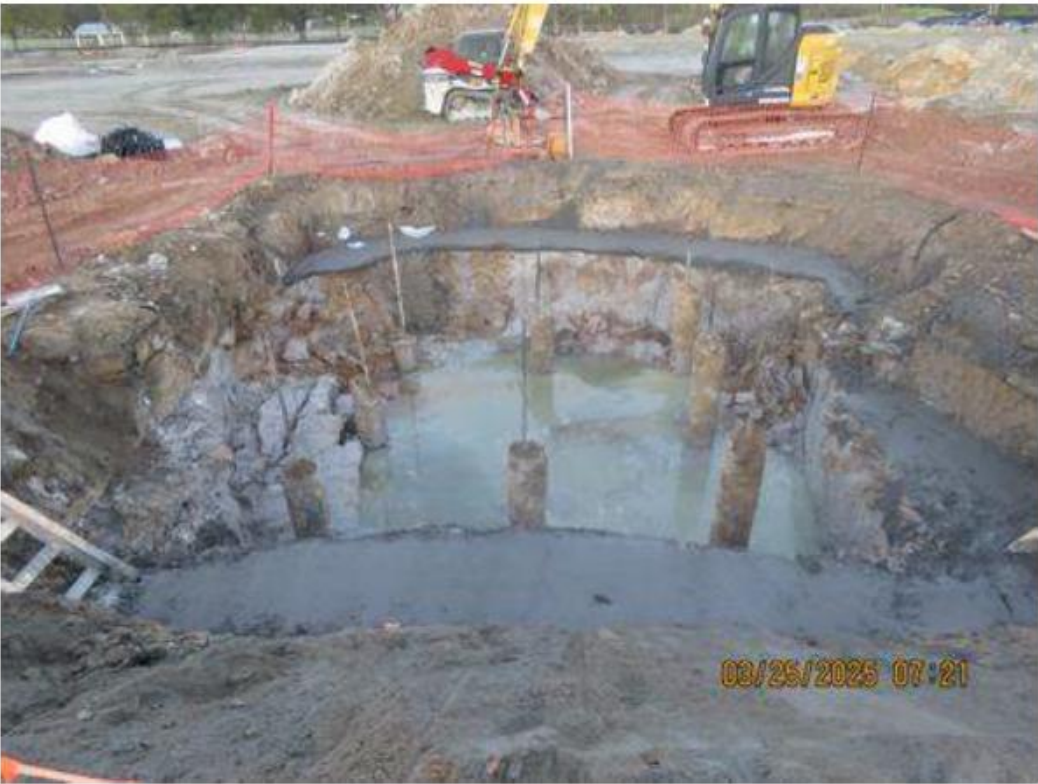
Tower crane foundation excavation and mud mat (water is ground water seepage)
