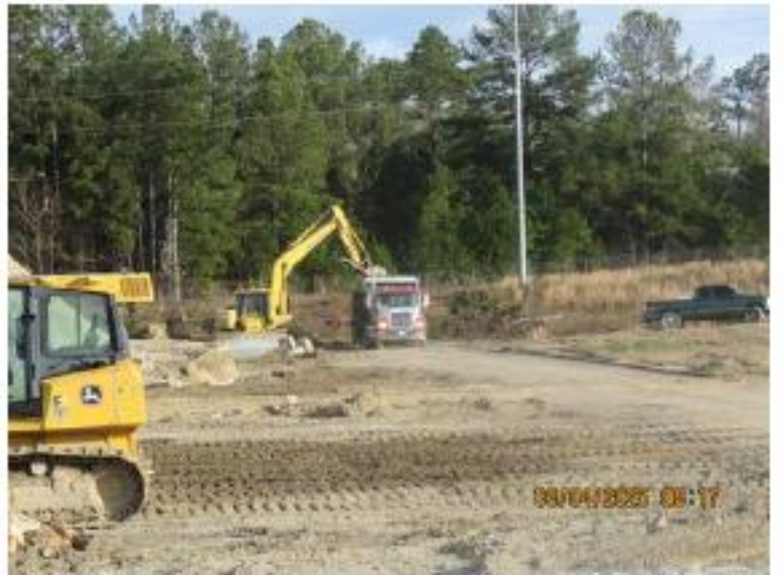
Carolina Power Starting Temp. Power
